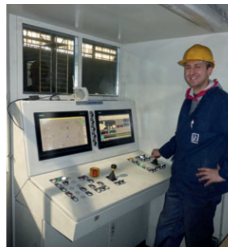
Operator control desk of pouring furnace
